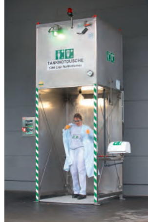
Tanknotduschen Tank safety showers
